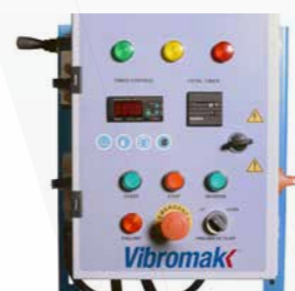
Electrical Control Panel
